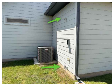
Vent and TR drain – left side
