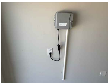
Irrigation controller – garage
