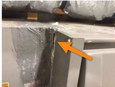
Supply Plenum connection
