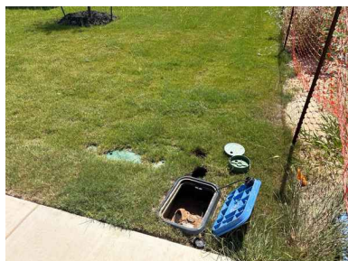
Water meter, supply valve, pressure reducing valve overview
