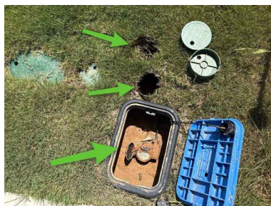
Water meter, supply valve, pressure reducing valve
