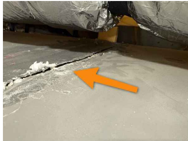
Supply Plenum connection
