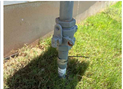
Shut off valve at meter
