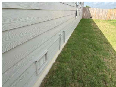
TPR and overflow drain – right side
