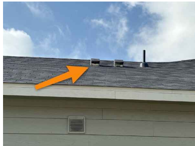
Dryer vent – right side
