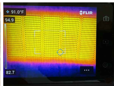
Example of fresh air makeup unit temperature reading at front hallway
