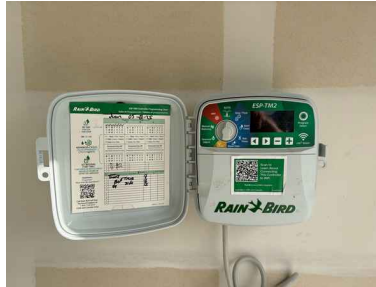
Irrigation controller – garage
