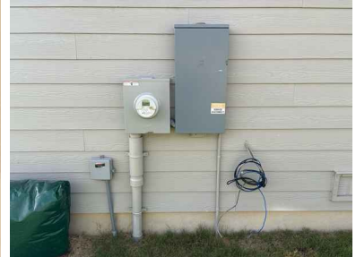
Electrical service entrance – right side
