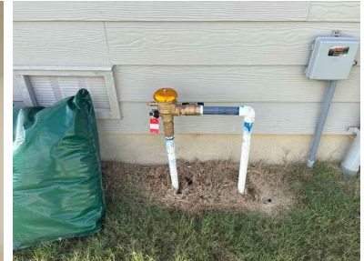
Irrigation backflow, and shut off valve – right side
