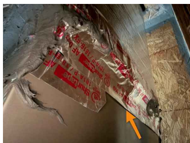
Backside of HVAC supply Plenum
