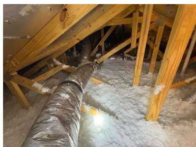
Fresh air makeup unit ductwork
